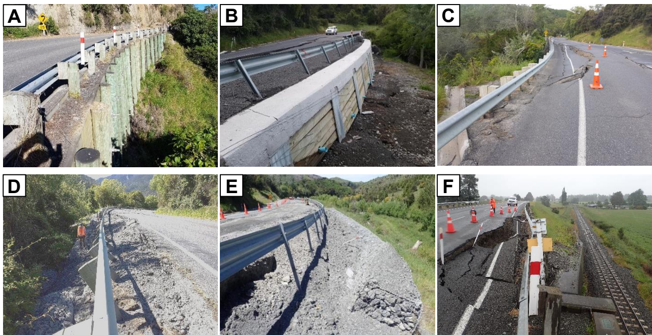
Figure 34: Examples of damage to retaining walls.
