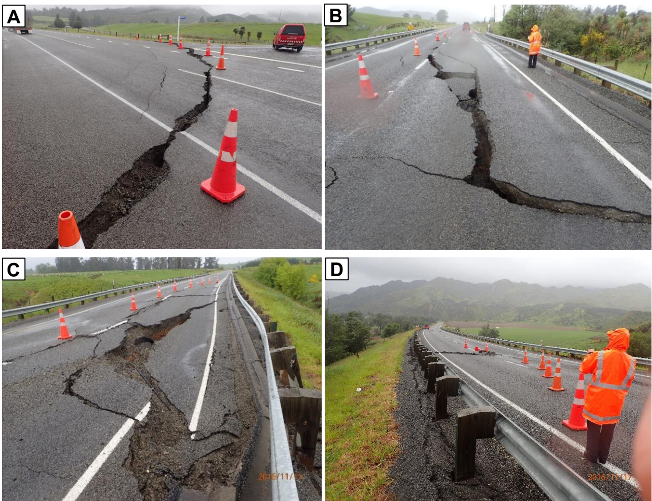
Figure 24: Damage to fill embankments on the Hawkswood to Ferniehurst section of SH1. (A) Hawkswood Stream; (B) Homestead Creek; (C) Culvert 55; (D) Chilly Stream. Photo credits: C. Parkes.
